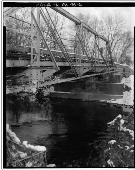
Eyebars in a Truss: The Washingtonville Bridge , Historic American Engineering Record, Photograph of a bridge built in the 1800s · Photograph · Library of Congress, Prints and Photographs Division
