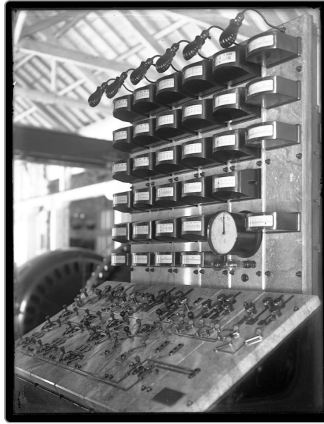
A Power-Plant Switchboard , Unknown photographer, about 1910 · Photograph · Possibly the Cedar Falls hydroelectric plant, Washington
